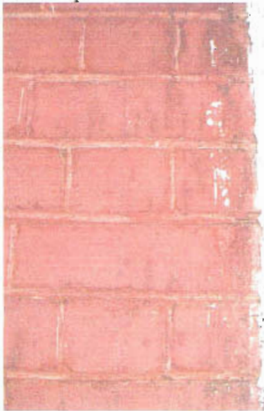
Paint drips on brick at Pavilion VIII
